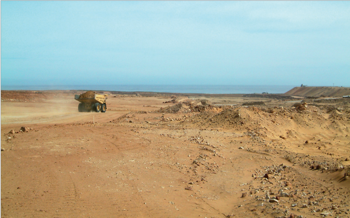
Figure 36: HM mining operation by Namakwa Sands with the Atlantic Ocean in the distance. Photo: DERA.
