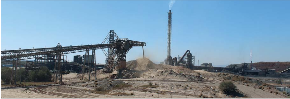
Fig. 3.13: Processing plant (crushing, milling) of the magnetite ore at the Rhovan plant (photo: DERA 2015).
