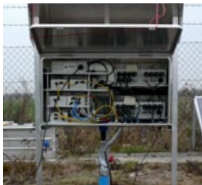
Installed monitoring station.
