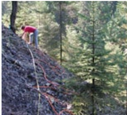
Installing electrodes for a geophysical survey of a mining heap in the western Harz.
