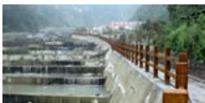
▲ Safety measures in China for protection against mudslides after the 2008 Wenchuan earthquake.
