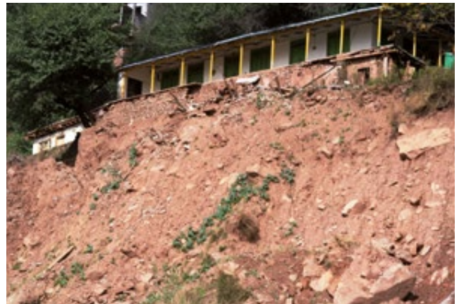
▲ A house destroyed by a landslide on the road from Islamabad to Muzaffarabad in Pakistan.
