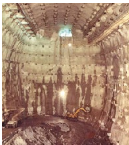
▲ Machine cavern during excavation with a combined lining with reinforced shotcrete and system anchors.
