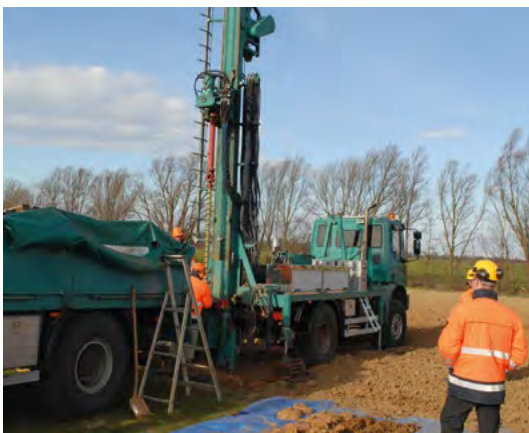
▲ Drilling in the field to obtain soil cores from the entire unsaturated zone.
