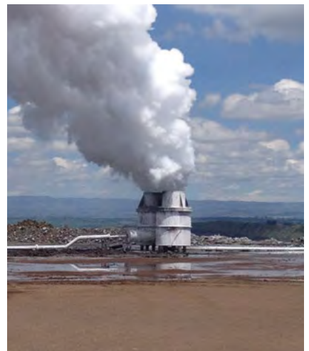
▲ Reservoir test of a new well in the Menengai field in Kenya.
