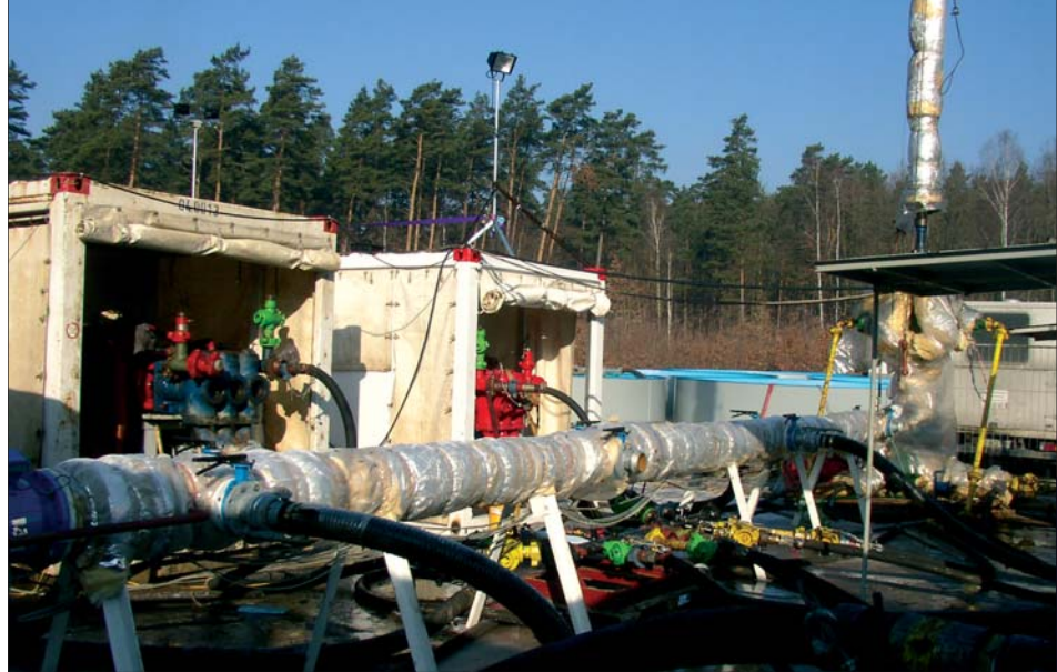
High pressure pumps, suction manifold and well head during the stimulation tests at the Groß Schönebeck borehole in January/February 2003.
