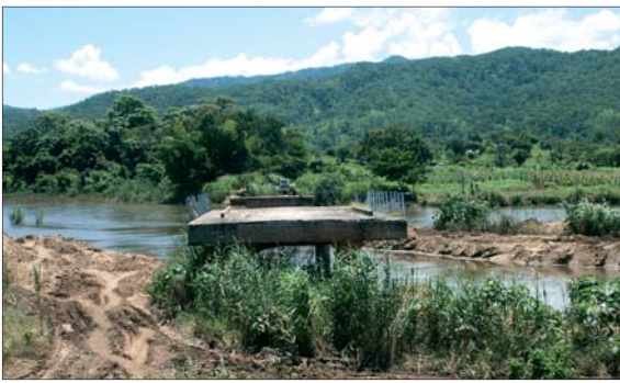
Dwambadzi River bridge: Remains of the bridge swept away by floods in 1999.
