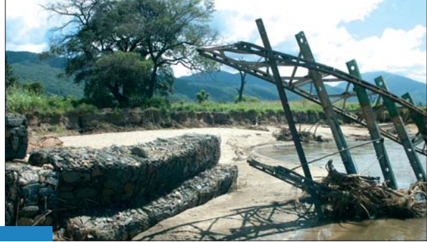
Dwambadzi River: Destroyed auxiliary bridge in 2001.
