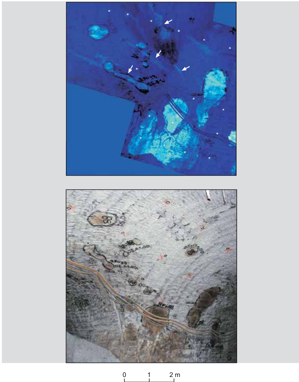
Figure 49: Condensate occurrence in cross-cut 1 West at the pillar corner of drilling location 1.4 at approx. drift metre 325 under ultraviolet light (above) and artificial light (below). The two photographs show the same area. The visible condensate inflows are marked by brown stains on the sidewall. Weak lines of fluorescence can be seen under ultraviolet light in the upper part of the picture corresponding to convergence-induced cracks originating from the corner of the pillar. These cracks release intercrystalline-bound condensates.
