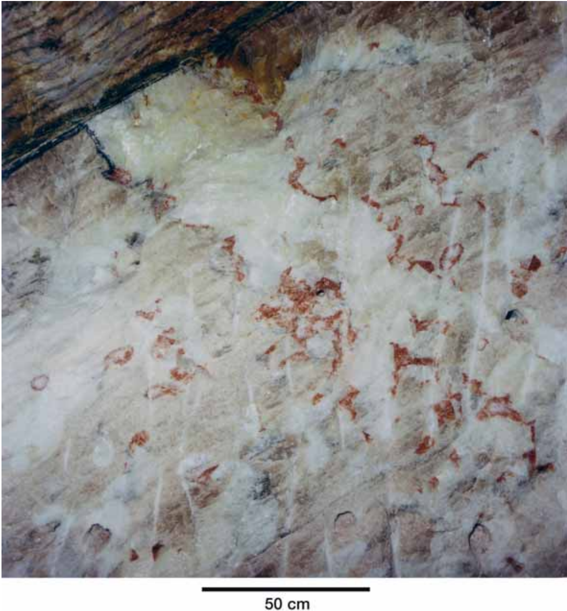
Figure 26: Starting at the Gorleben-Bank, a secondary mineralization permeates the underlying Unteres Orangesalz, the sedimentary bedding of which is almost completely destroyed in this area. No fault-induced dislocation of the bedding is detectable. The mineralization consists mainly of white coarse-crystalline halite and red carnallite on the edges. Milling workshop, 840 m-level, drift position 65 m. (Photograph: Bauer, DBE)
