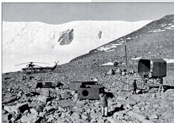
Construction of the "Lillie Marleen Hut" in a rocky depression next to the Lillie Glacier
