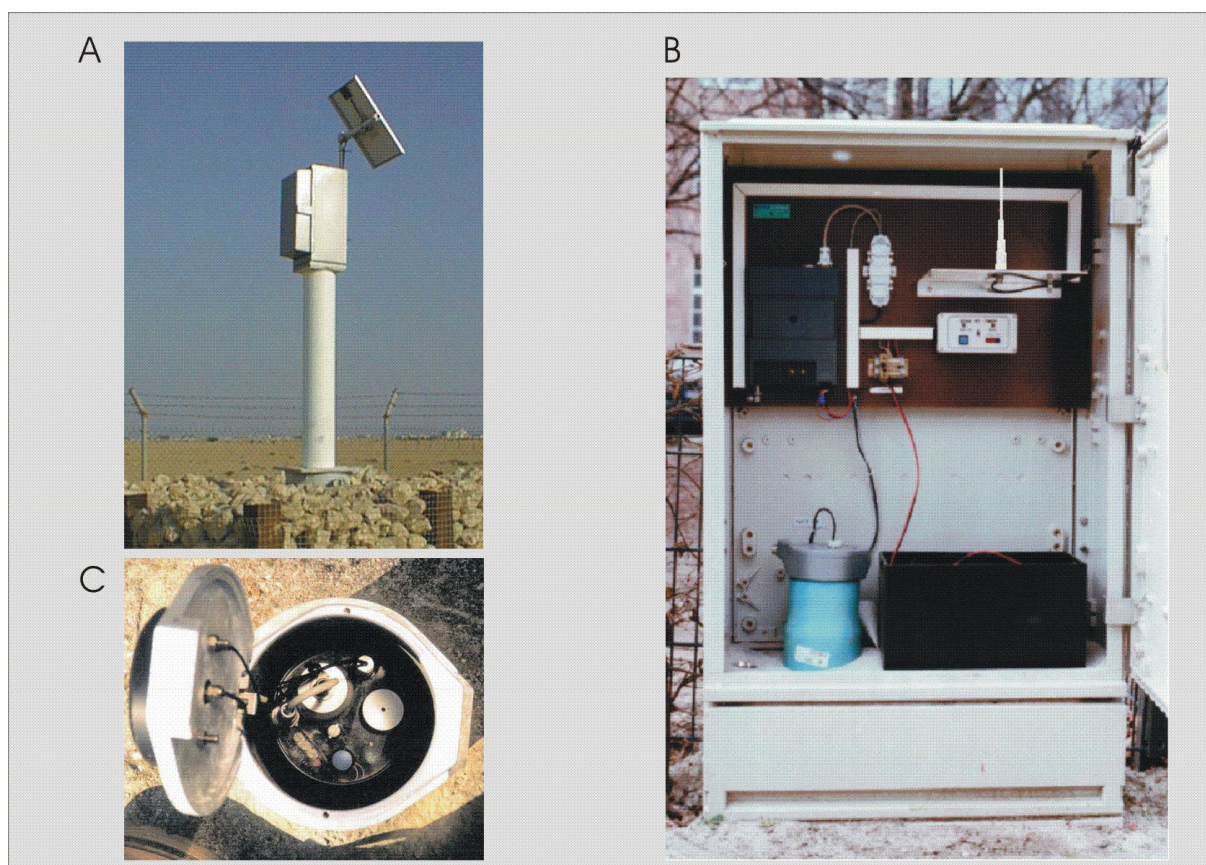
Figure 6: Examples of Telemetric Data Transfer from Groundwater Monitoring Stations using a) GSM Data Transfer in Combination with a Solar Panel, b) Radio Signals; Power supplied by the Local Power Grid or c) GSM Data Transfer in Combination with Standard Battery Packs (Courtesy SEBA)
