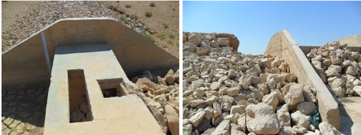
Fig. 14: Wadi Madoneh: left) dam M2: metal parts from gabions and manhole were stolen and release pipe opening/closing mechanism blocked with large stone, right) dam M1: damage to dam due to the use of material not adhering to the specifications (Picture taken by A. Steinel in 2011).
