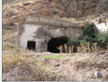
Residues of former mining activities
