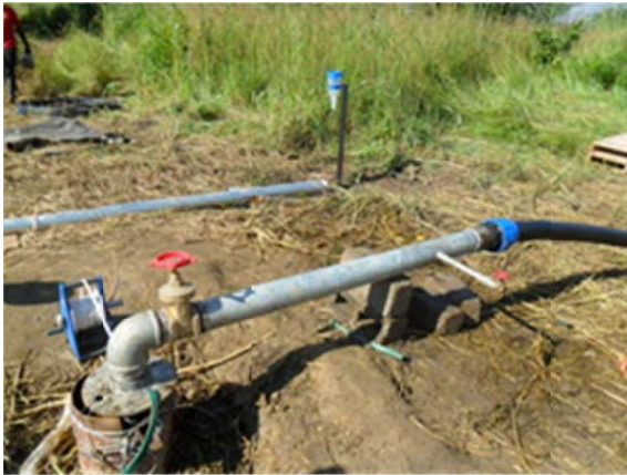
Figure 7: 4” discharge pipe at well head
