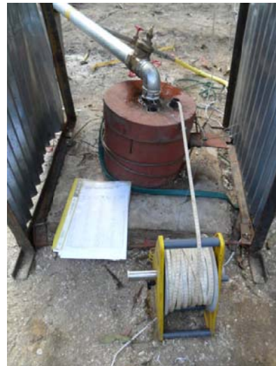
Figure 10: 2” discharge pipe at well head
