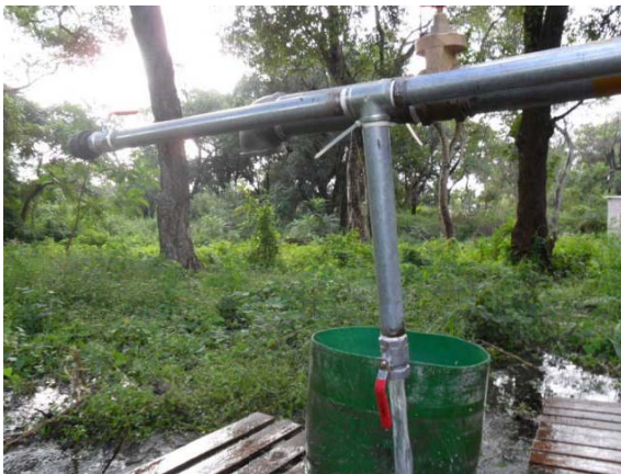
Figure 9: 2” discharge pipe at discharge point
