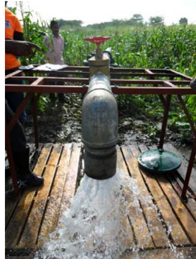
Figure 8: 4” discharge pipe at discharge point
