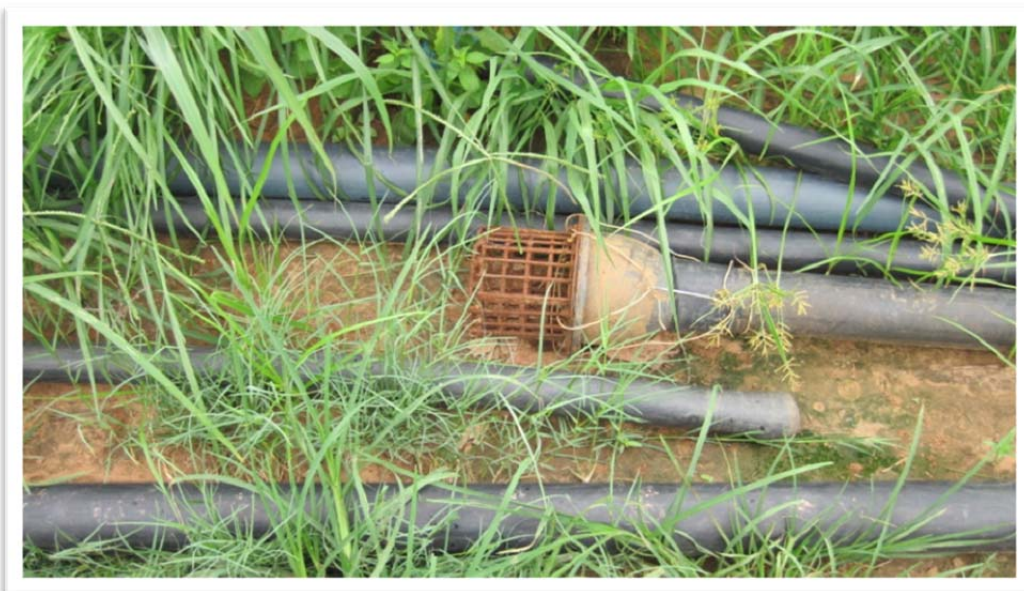
Figure 6 Intake pipes for water abstraction
