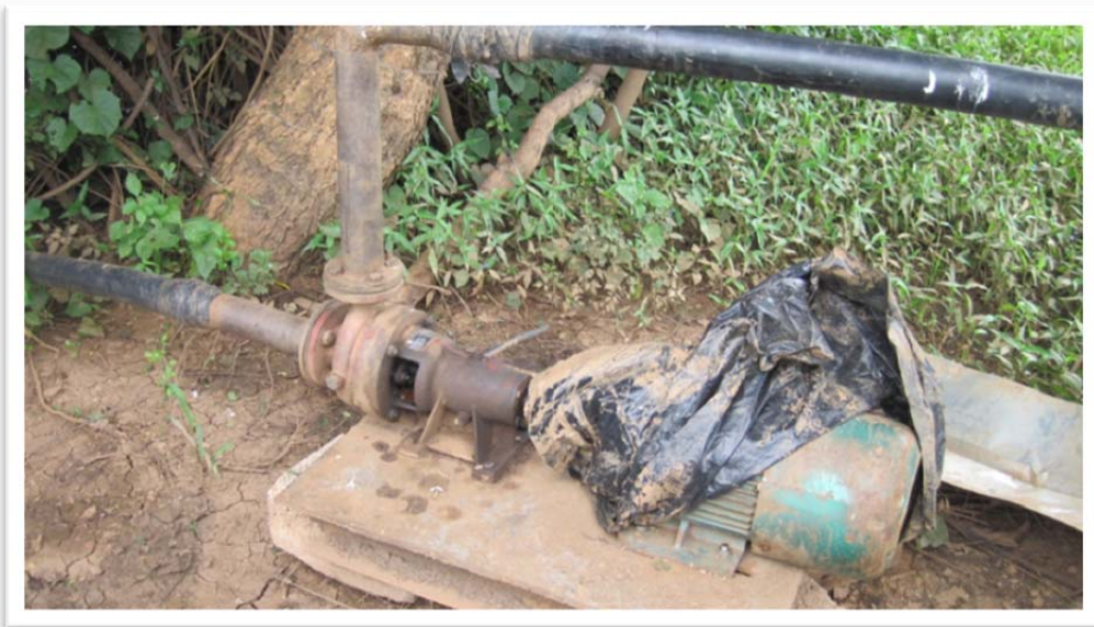
Figure 5 A small pump used to abstract water from the Chongwe river
