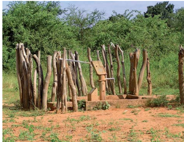
Handpump, type India Mark II.
