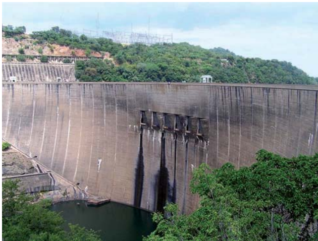
The Kariba dam wall was built into an intrusion of granitic gneiss near Siavonga into which the Zambezi has incised a deep gorge.
