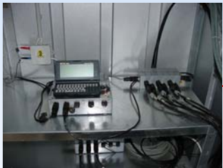
Control panel (TDR)
