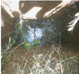
Incomplete pit latrine hole with water
