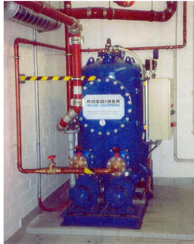
Vacuum station (pump) 08
