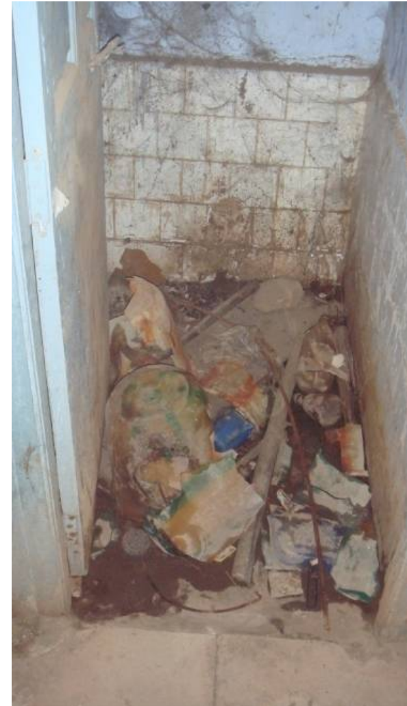
Existing toilets are in bad condition
