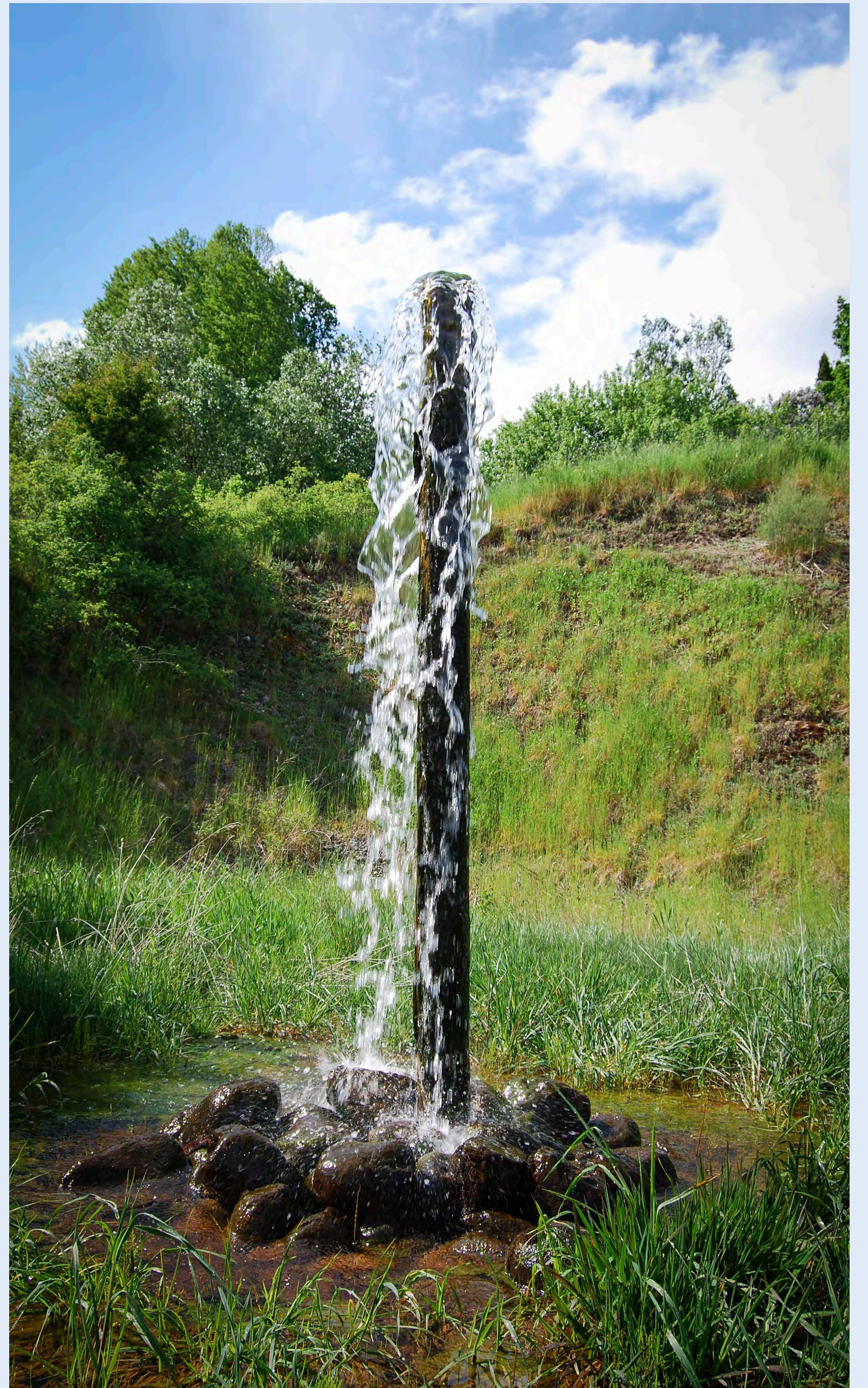
Aeration of a groundwater supply well. Photo: Magdalena Thorsbrink.
